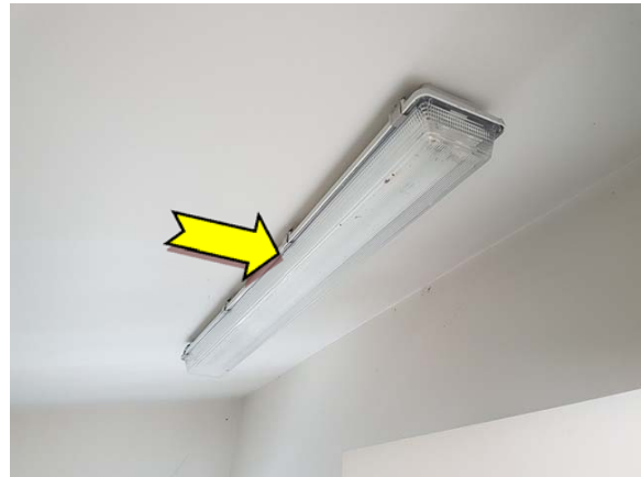
Photo 4. Interior, throughout, double tubed fluorescent light fitting – suspected PCB-containing capacitors.
