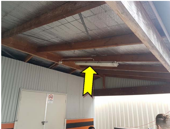
Photo 3. Exterior, throughout, double tubed fluorescent light fitting – suspected PCB-containing capacitors.
