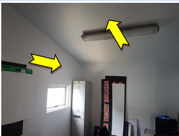
Photo 5. Interior, throughout, walls and ceiling – suspected lead-containing white upper paint systems.
